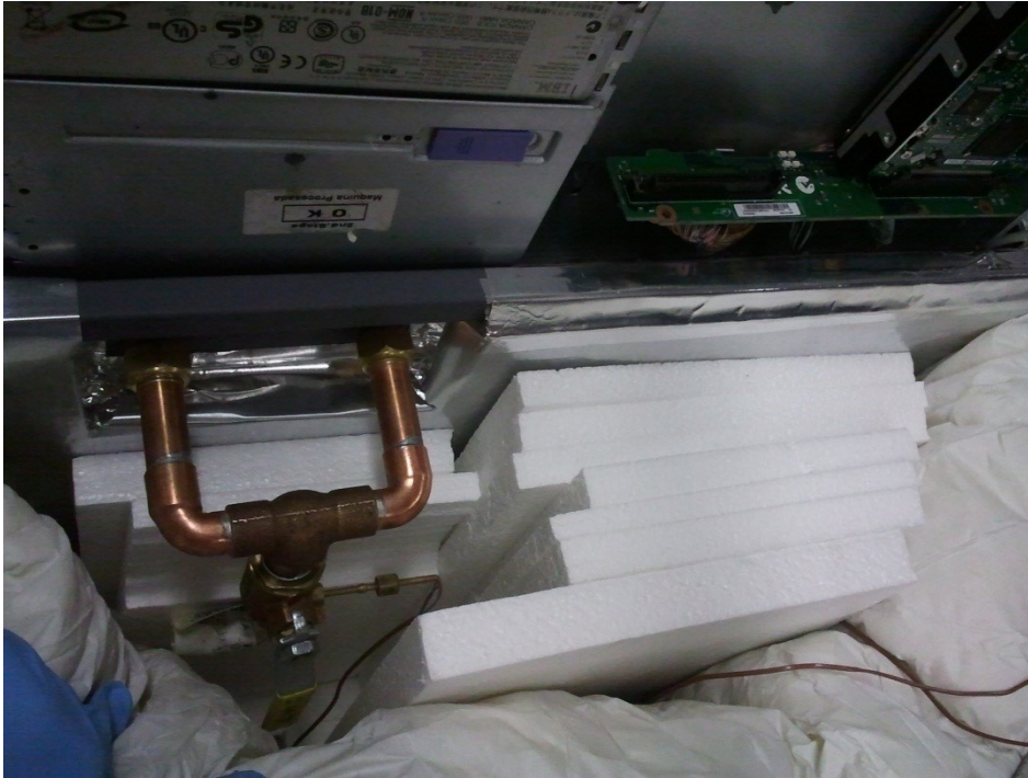
Figure 19. Manifold fitted over CPUs is used to direct the highest quality thermal energy (i.e., high temperature heat) into the discharge line and ideally to an absorption chiller. The differential thermocouple plumbed into fitting gauges the discharge temperature. The remaining heat supplied by 1U IBM eServer xSeries 336 server blade is transferred into the clear, odorless, non-toxic, dielectric, technical grade white mineral oil optimized for cooling servers and other data center hardware.
