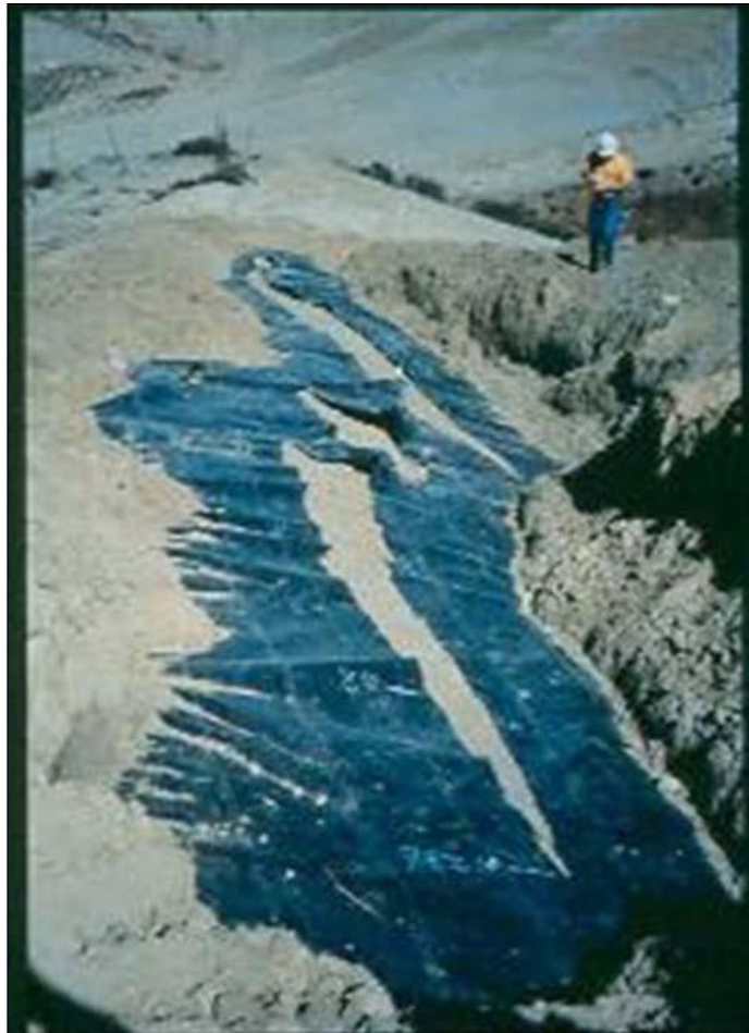
Figure 1-2. Tear in geomembrane liner system, Cell C, Chiquita Canyon Landfill after 1994 Northridge earthquake (photo courtesy of Calif. EPA, Integrated Waste Management Board)
