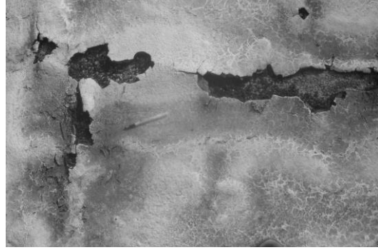
Fig. 2: Defective SPF roof with open
