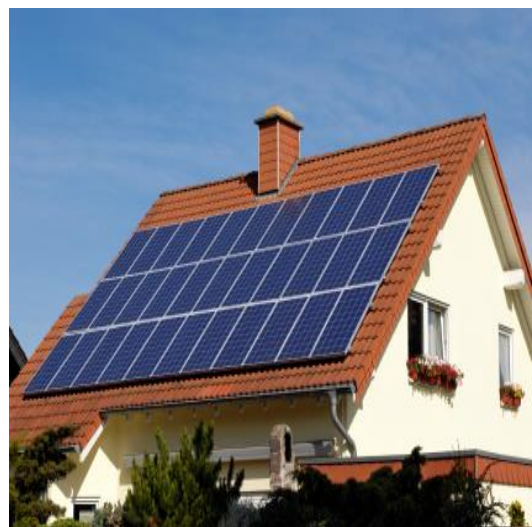
FIGURE 32. SOLAR PANELS ON A GABLE
