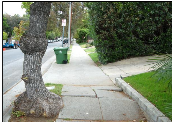
FIGURE 8. DESTROYED PAVED SURFACE BY TREE ROOTS. PHOTO CREDIT: IAN LOVETT
