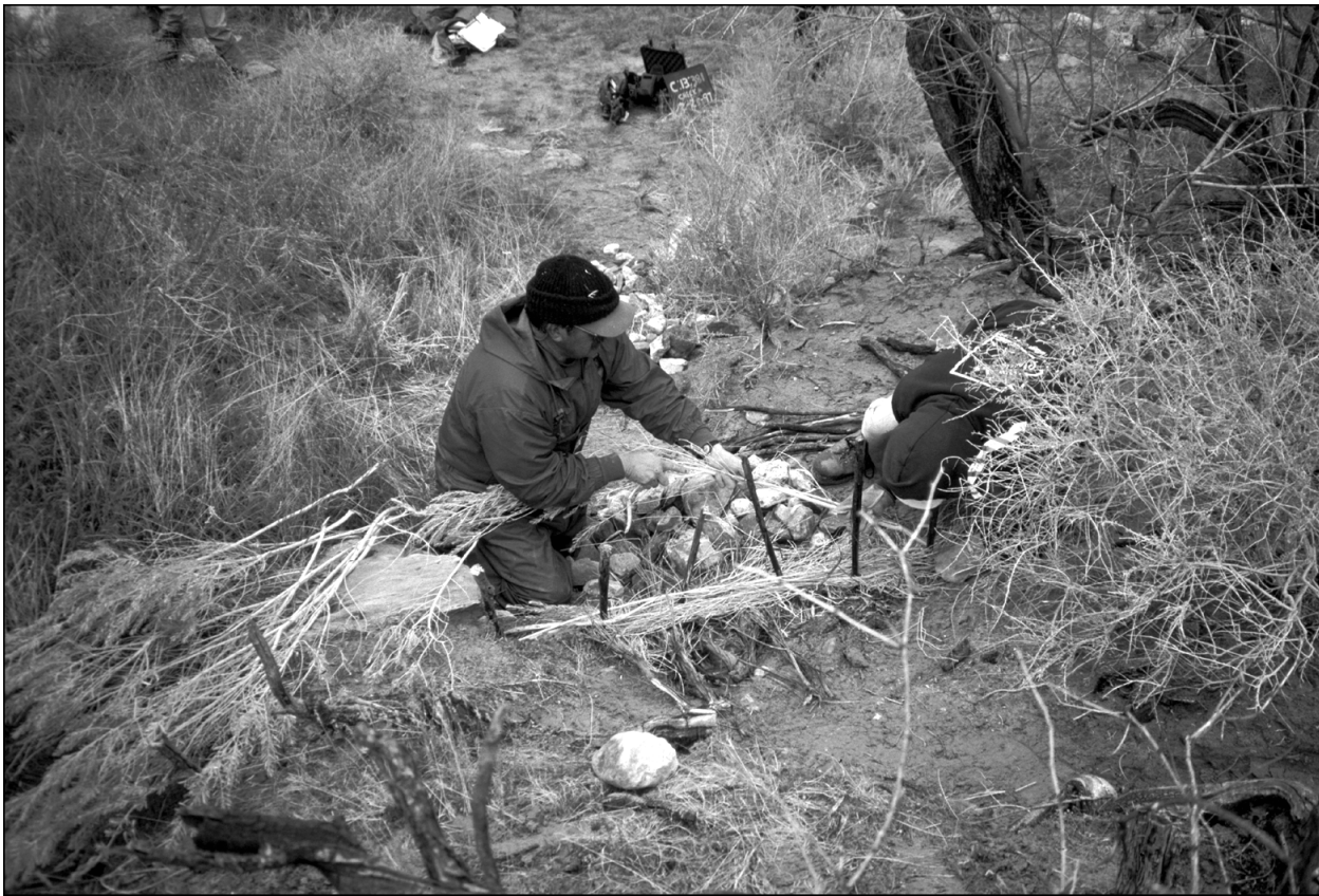
Figure 33. Soil conservation specialists from the Pueblo of Zuni installing erosion-control checkdams at site AZ C:13:381 (courtesy of Grand Canyon National Park Archaeology Program).
